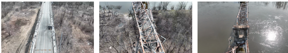
Fig. 4. Examples of drone imagery for Chernihiv Bridge, damage level 'mixed'.
